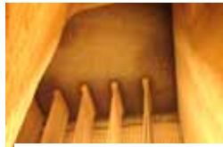
燃焼室天井 MUC - SC80 RSC - 60WG
